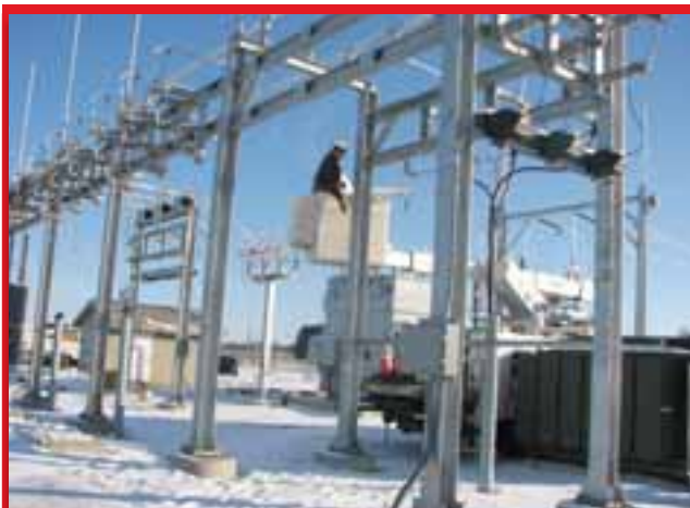
The new Red Hawk Substation will serve the increasing demand for electricity in the Milton Township area and support anticipated growth of the Milton Crossroads Business Park.
