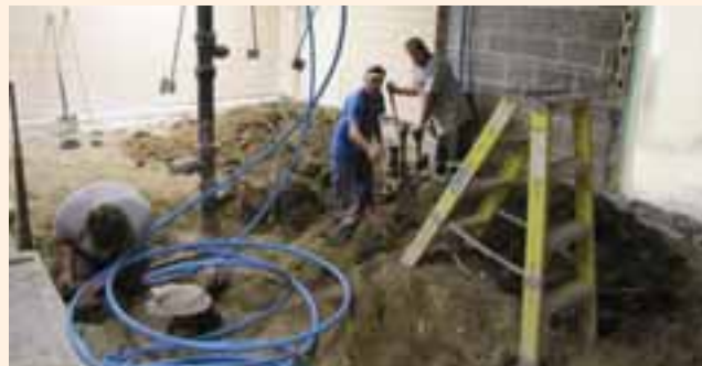
Workers from Ladage Construction and Snell Plumbing install new piping for the restrooms at Rural Electric's office. New concrete floors were poured in late October. (The space shown will include both the men's and women's restrooms.)
