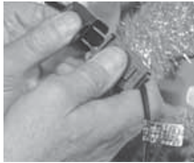
Check to make sure connections are secure and cords are not worn or frayed. Source: Underwriters Laboratories (UL)
