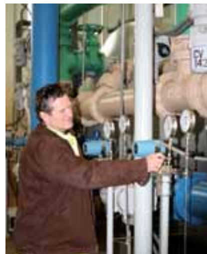
Water Superintendent Dave Troxell checks a gauge at one of the Petersburg Water Treatment Plant's filters, also shown below.
