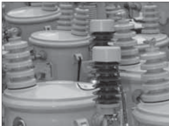
Thieves across the country are damaging electrical equipment like these transformers for the copper they contain. Some thieves are paying for the theft with their lives.
