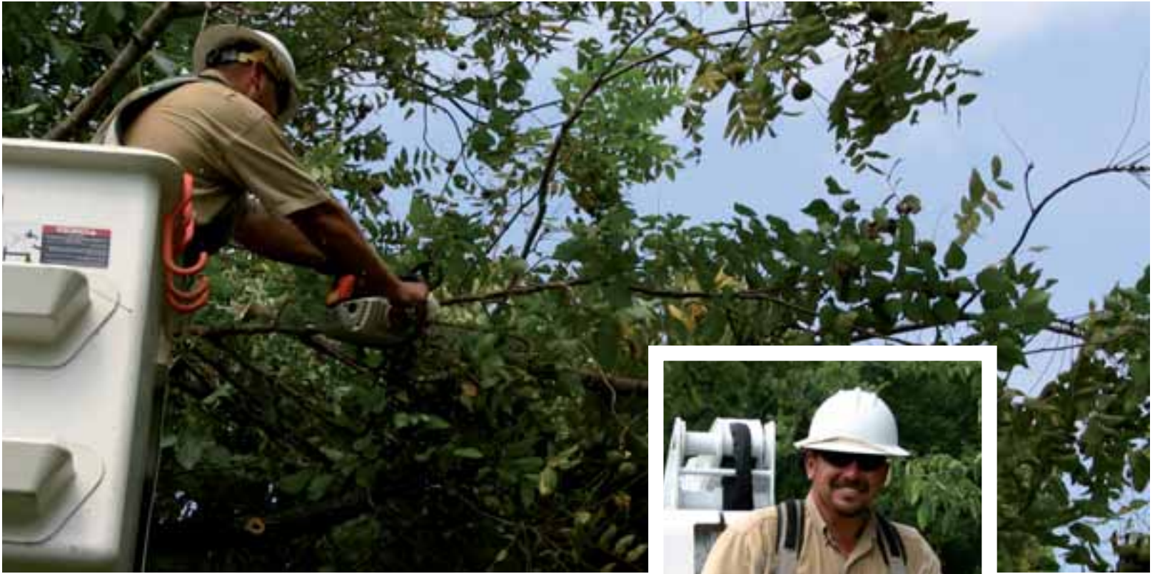
Darren Hayn trims back a tree that is too close to a power line.
