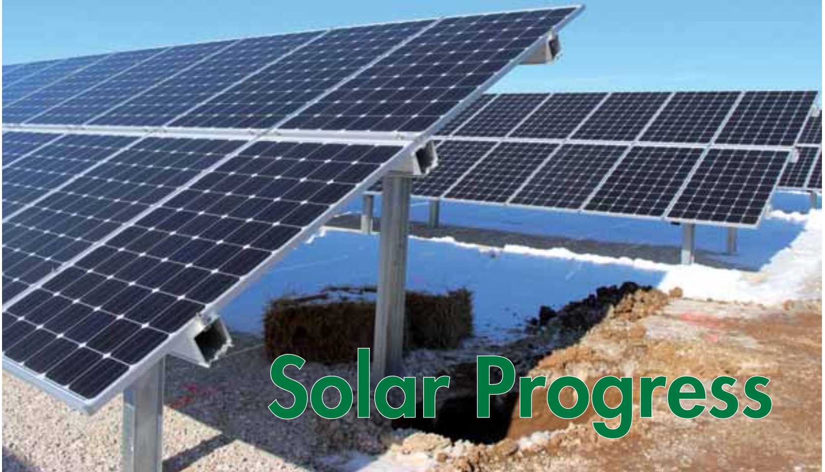
Installed solar panels at the Scott County Solar Plant between Winchester and Alsey.
