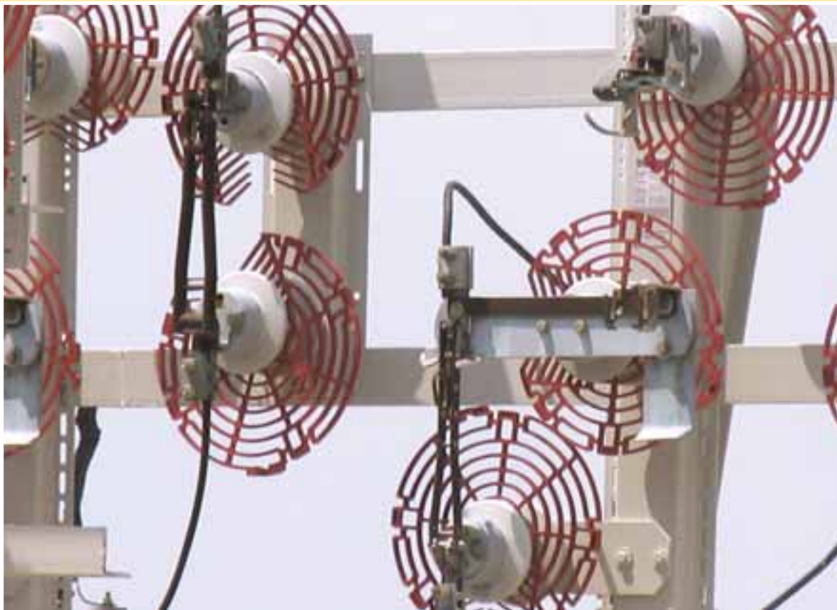
Squirrels and raccoons can cause blinking lights or power outages if they come in contact with energized wires on a pole or in a substation. Therefore, EnerStar installed wildlife guards in strategic locations within the Brocton substation.
