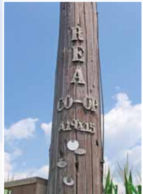
This old pole is still going strong! It is stamped with the REA information and the badges show the history of pole testing.
