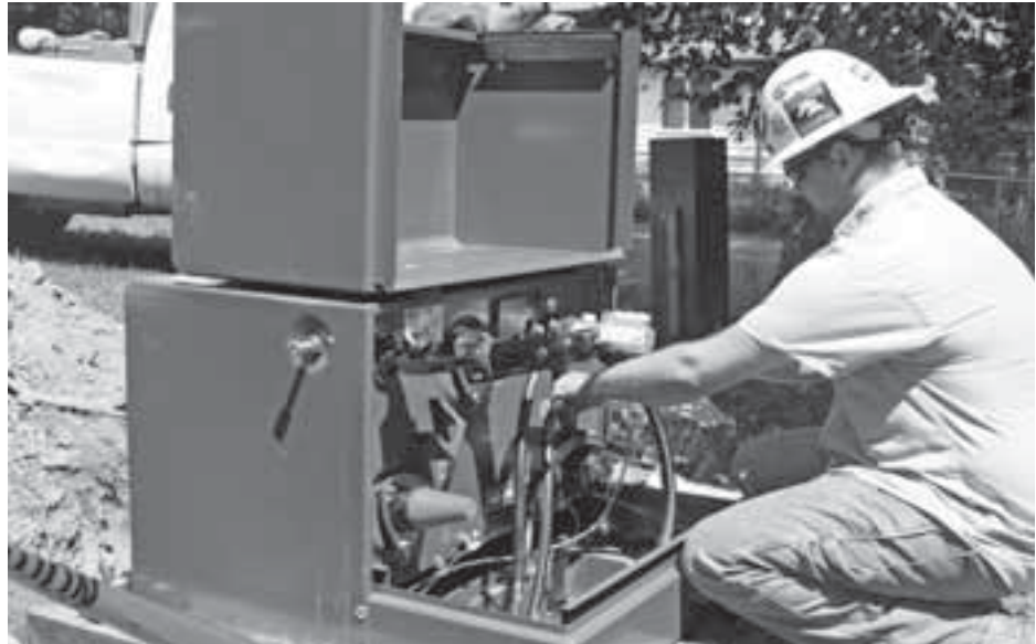
Lineman with contractor installing new underground cable makes connection to a new transformer in Parrish Acres west of Carbondale.
