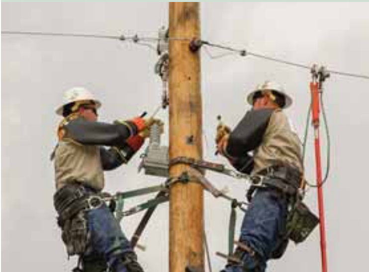
Left to Right: CCECI Apprentice Linemen Justin Hubert and Jacob Haselhorst can be seen here performing a single phase capacitor changeout.
