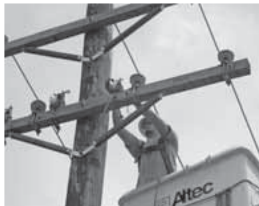
▲ Here a Big D Electric crew member is installing stringing pulleys to the newly constructed cross arm.
