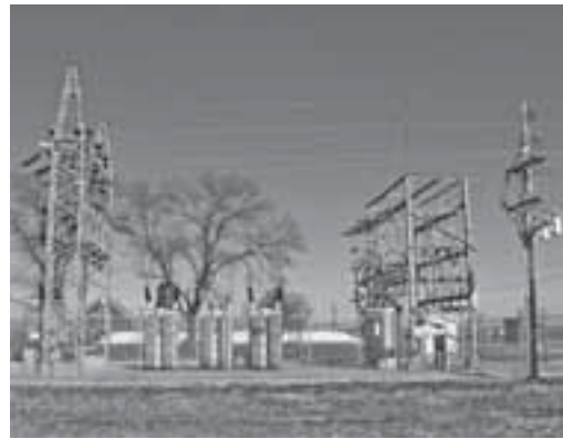
Our existing Ferrin Substation (May 2012)
