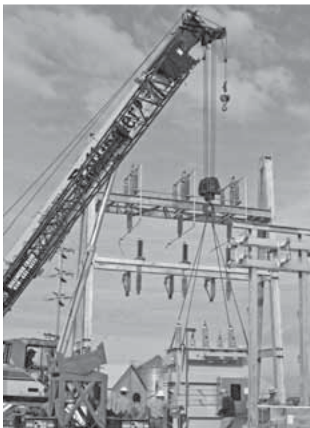
The transformer is carefully guided into place and strategically set onto its concrete foundation
