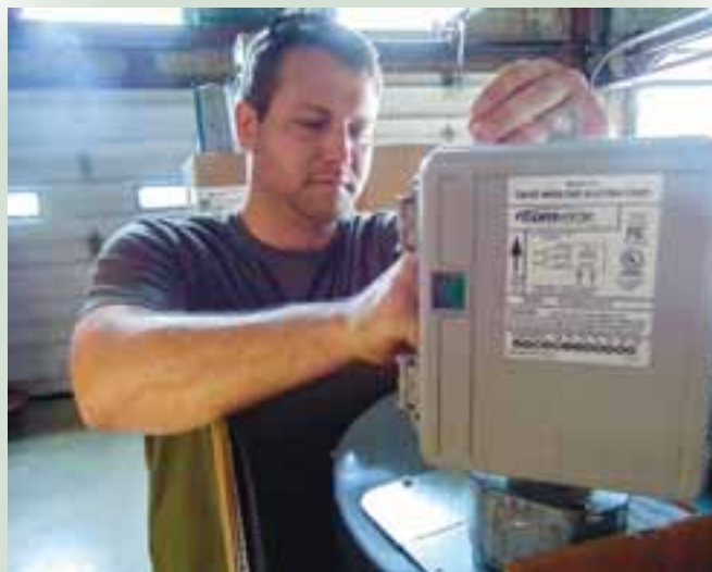
CMEC Marketing Services Specialist, Drew Haumesser, installs a load management device on a water heater. CMEC's water heater program has helped its members save money for over 24 years.
